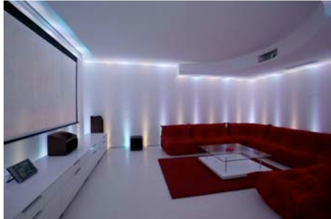
Home cinema with LED colour changing lights, recessed projector, screen, AMX Modero control and surround sound system.
